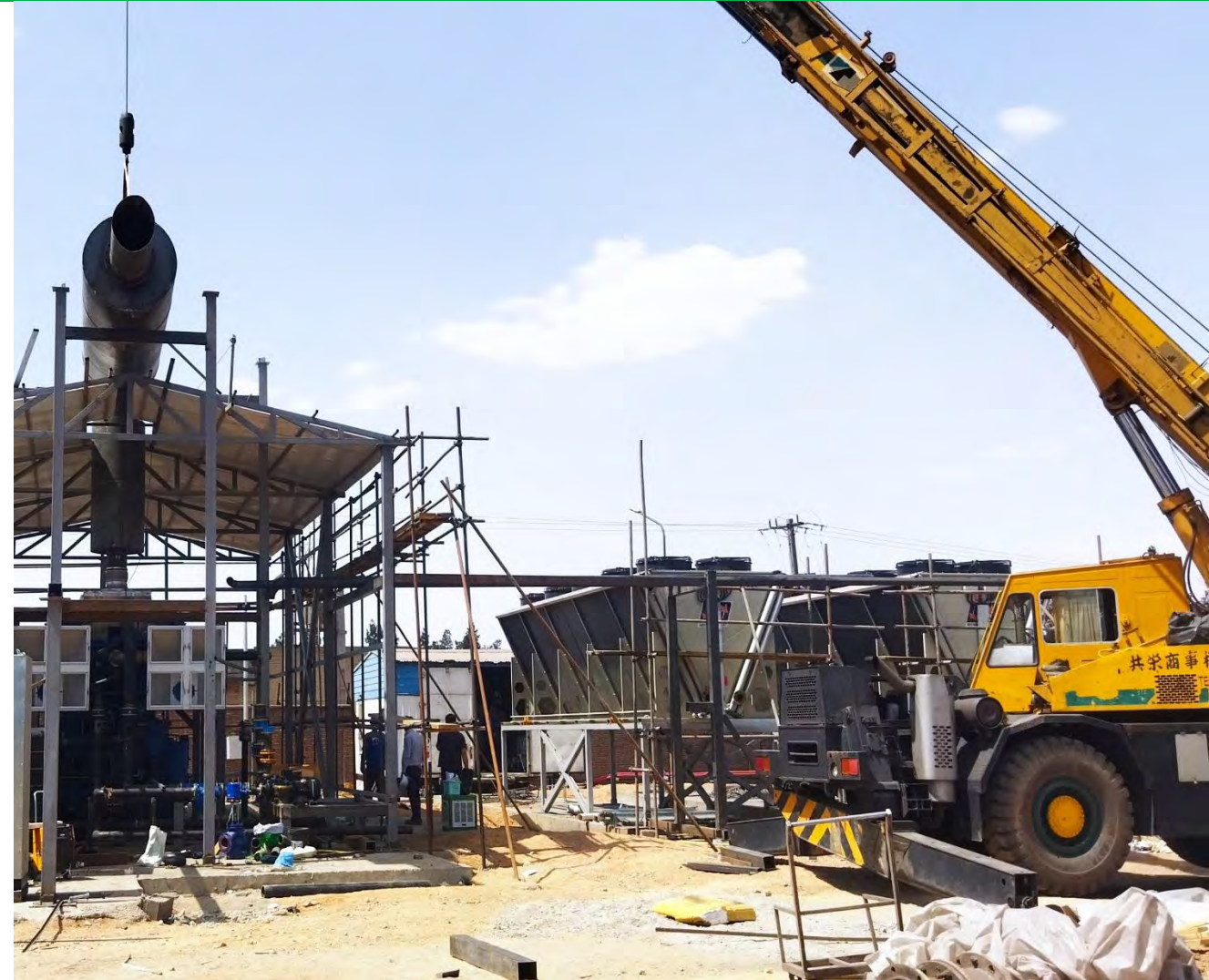
15 MW gas engine power plant of Golgohar complex
